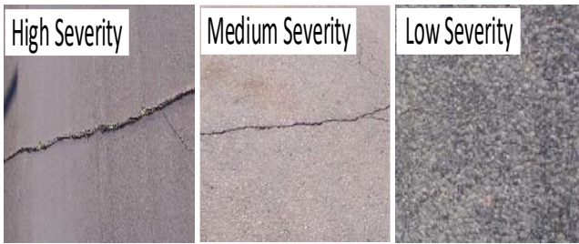
Figure. 10 Examples of different severity levels of transverse cracking
