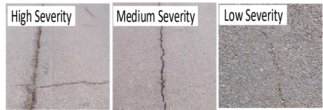
Figure. 11 Examples of different severity levels longitudinal cracks
