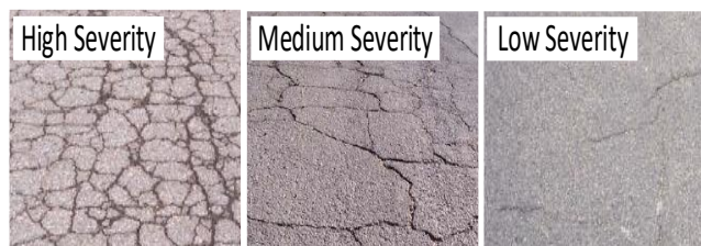
Figure. 9 Examples of different severity levels of alligator cracking
